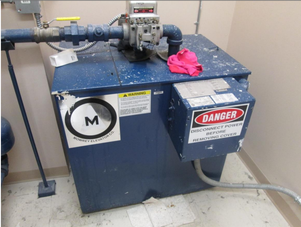
Photograph 9: Lazarra, 40 Gallon Reservoir Hydraulic Elevator
