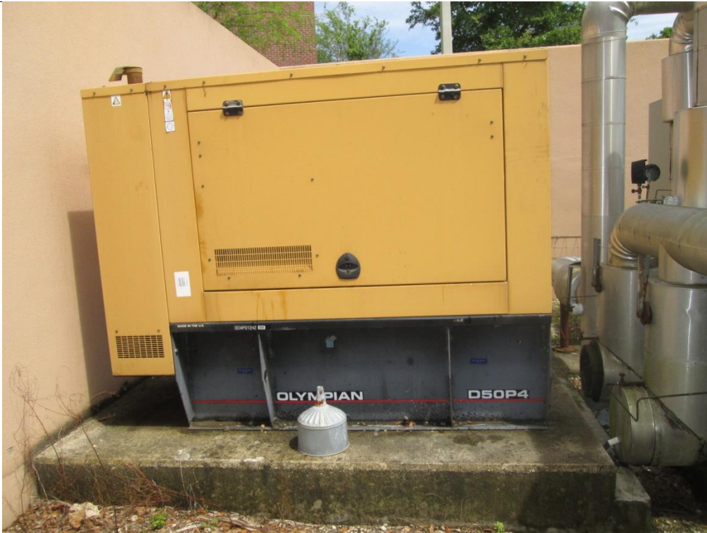
Photograph 14: Oak Hall, 160 Gallon Diesel Emergency Generator
