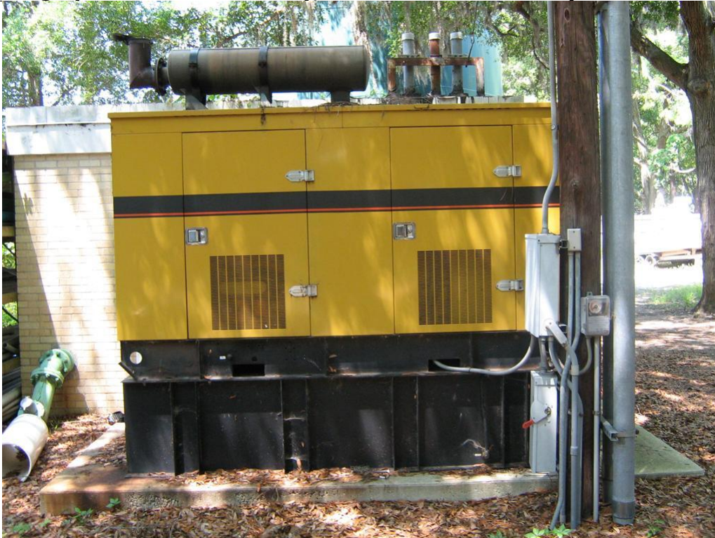
Photograph 22: Water Treatment Plant, Emergency Generator
