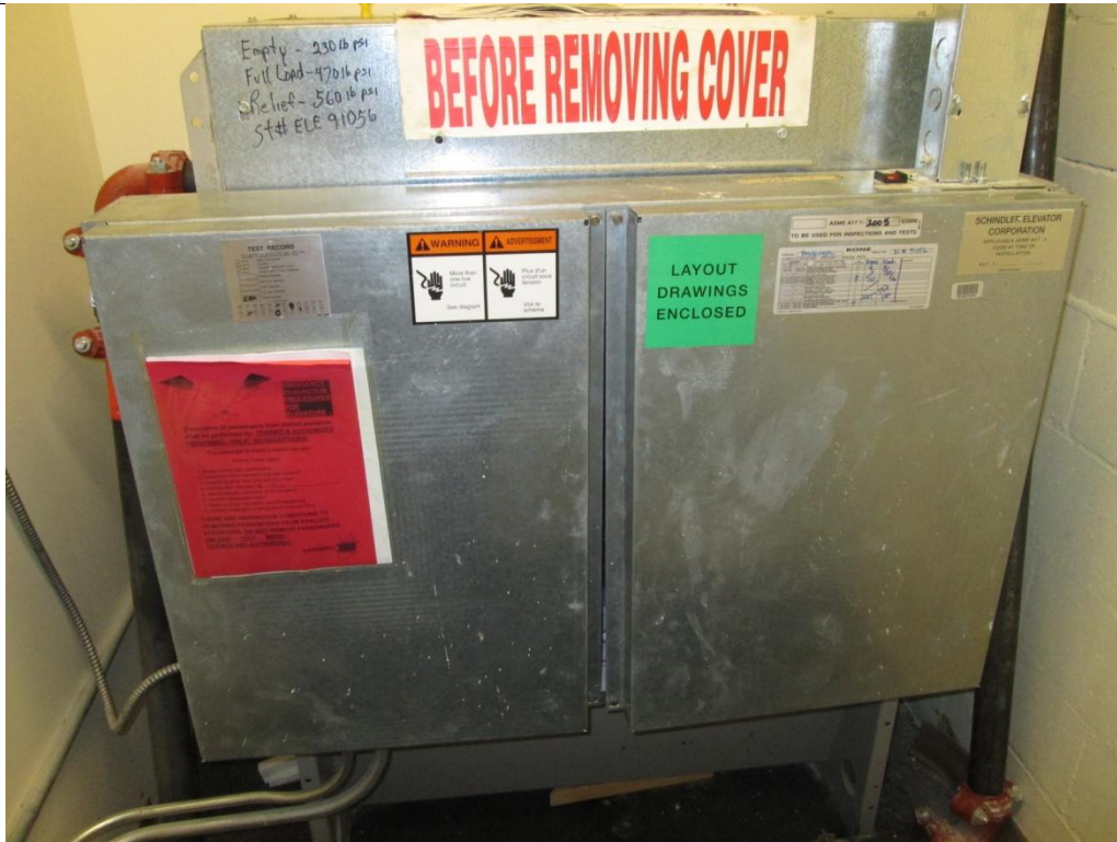
Photograph 20: Swisher Auditorium, 45 Gallon Reservoir Hydraulic Elevator
