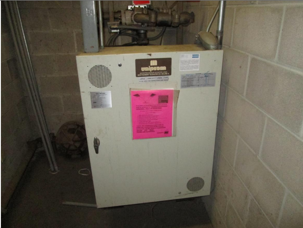
Photograph 3: Davis Student Commons, 90 Gallon Reservoir Hydraulic Elevator
