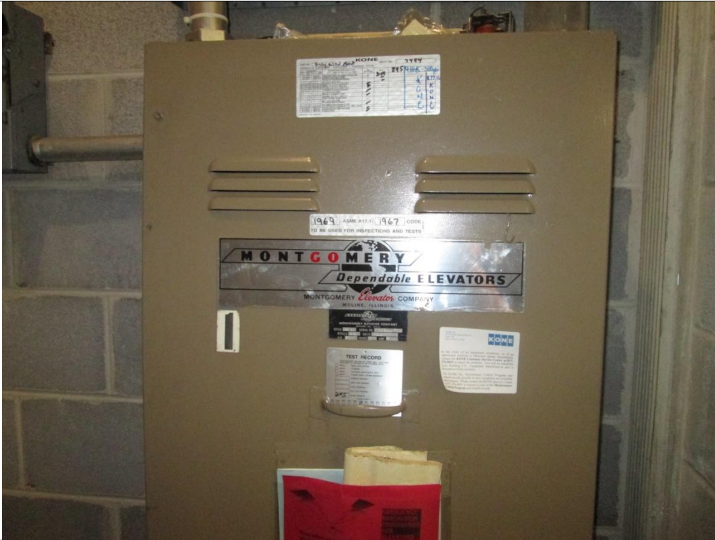
Photograph 21: Swisher Library, 100-Gallon Reservoir Hydraulic Elevator
