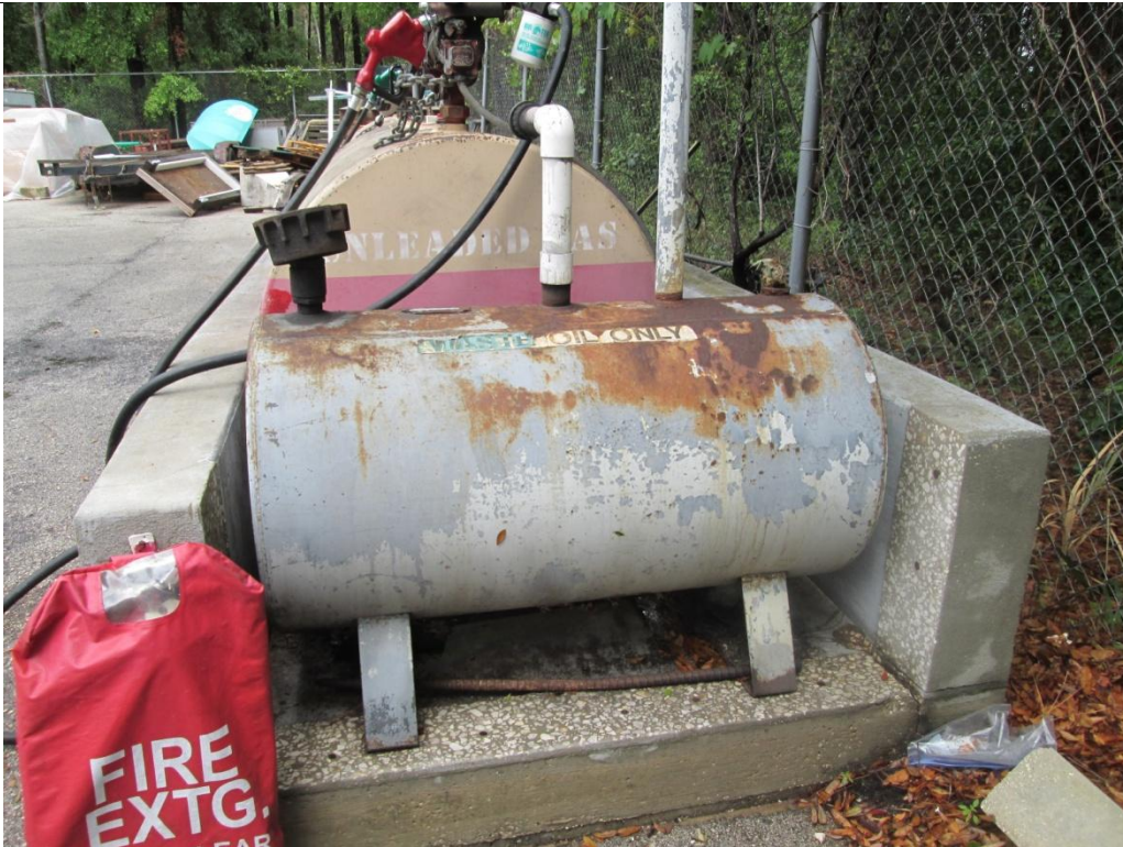
Photograph 16: Physical Plant, 250 Gallon Used Oil AST
