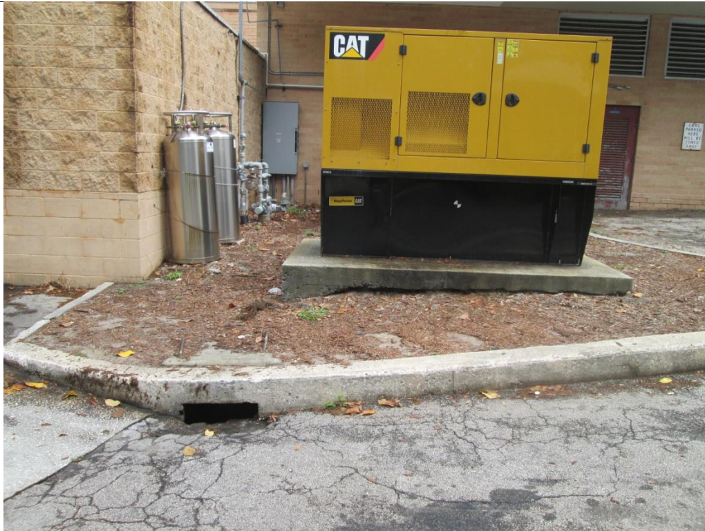
Photograph 8: Kinne University Center, 194 Gallon Diesel Emergency Generators
