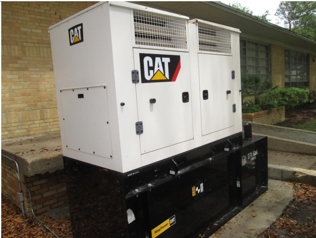
Photograph 4: Founders Hall, 271 Gallon Diesel Emergency Generator
