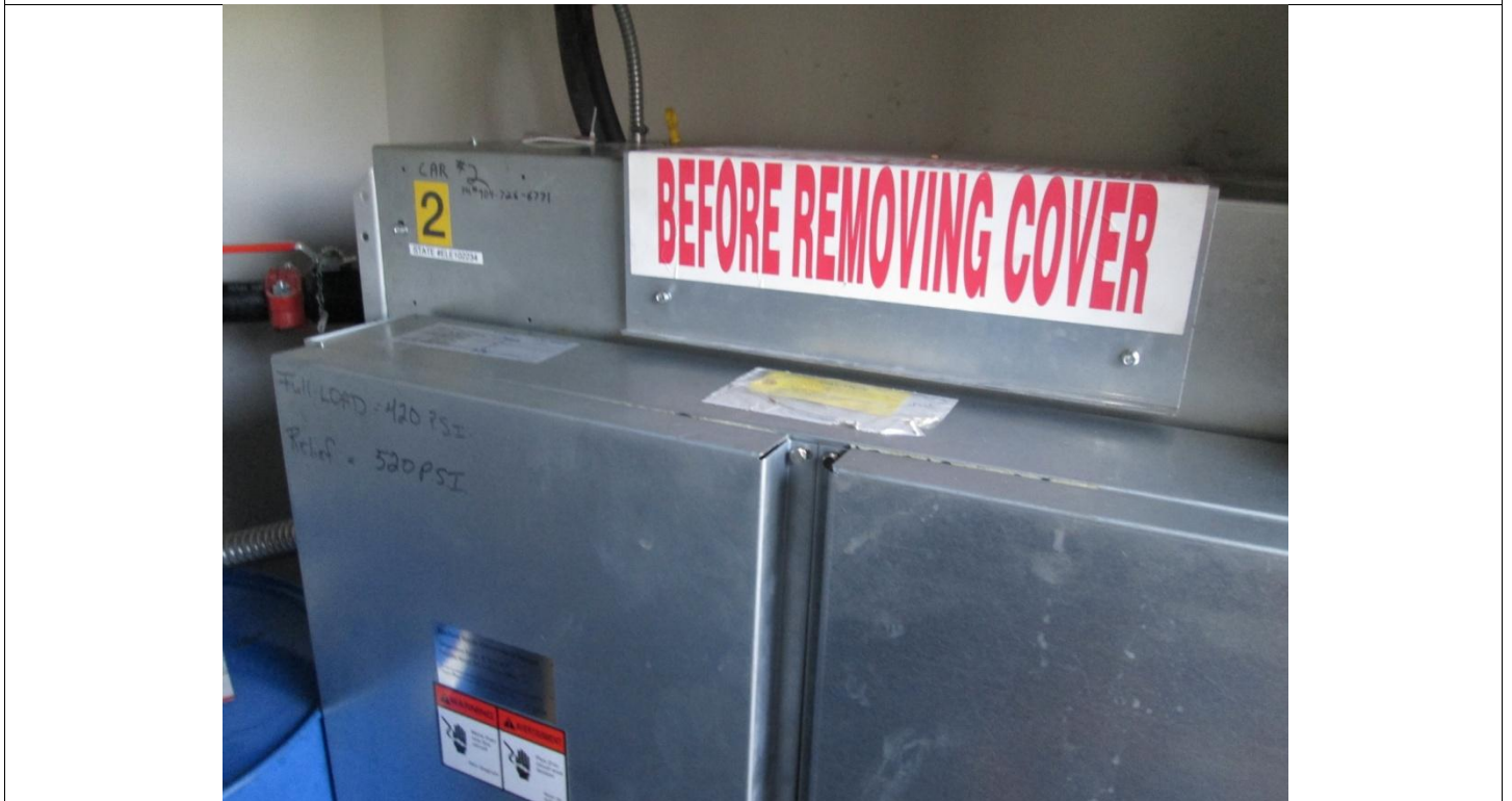
Photograph 12: North Hall #2, 60 Gallon Reservoir Hydraulic Elevator
