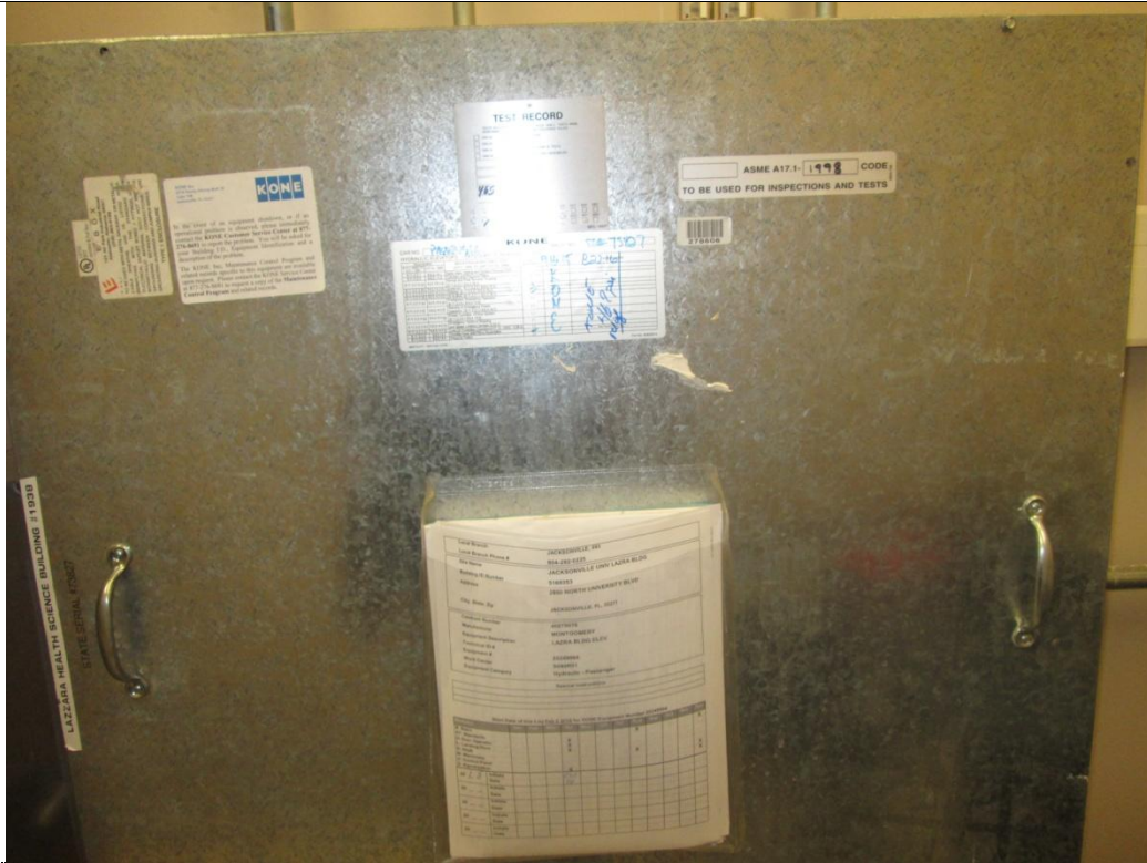
Photograph 19: Reid Medical Center, 65 Gallon Reservoir Hydraulic Elevator
