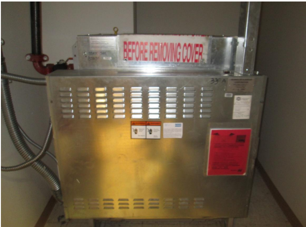
Photograph 2: Davis College of Business, 60-Gallon Reservoir Hydraulic Elevator
