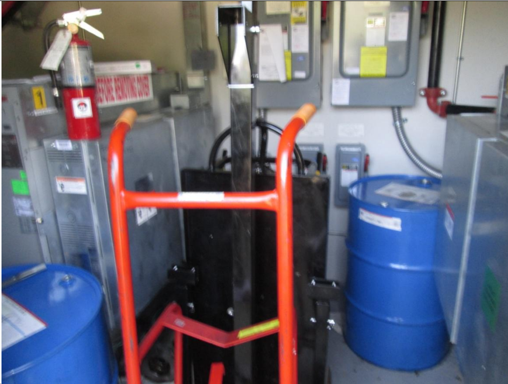
Photograph 13: North Hall #1, 60 Gallon Reservoir Hydraulic Elevator with Spill Kits
