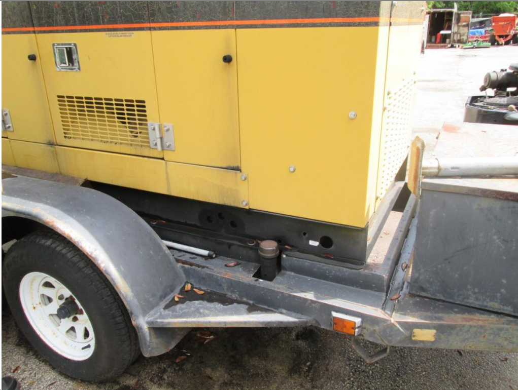
Photograph 15: Physical Plant, 60 Gallon Diesel Emergency Generator
